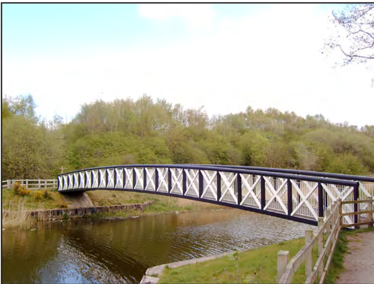
Fig 85: Carden's Ferry bridge over Witton Brook, connecting Anderton Nature Park to Carey Park.
